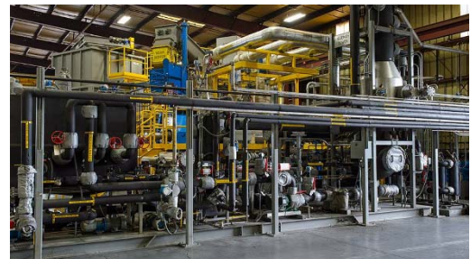
Photo 3: Plastics Pyrolysis Facility
